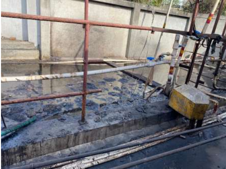
Collection tank of MVRE with floating sludge.
