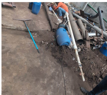
Underground tank behind MVRE (having outlet pump without any further fix pipeline system).
