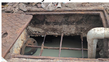
Underground tank behind MVRE (having whitish coloured contaminated water)
