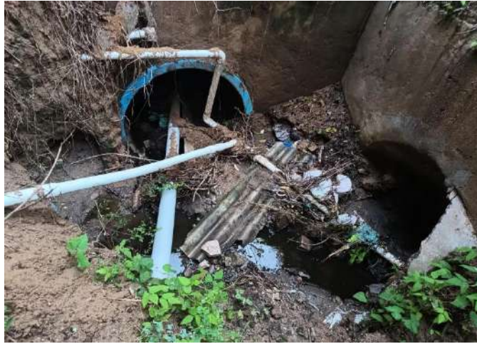
Contaminated water flowing into natural drain in front of unit.
