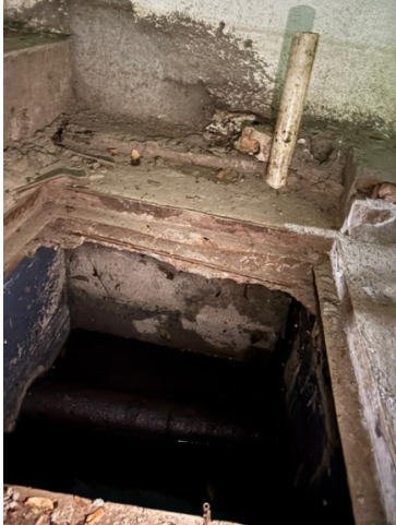
Storm water drain found seal
