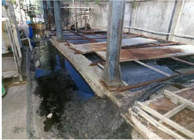
ETP tanks found full up to brim level
