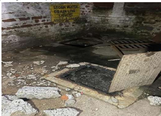
Overflowing of septic tank
