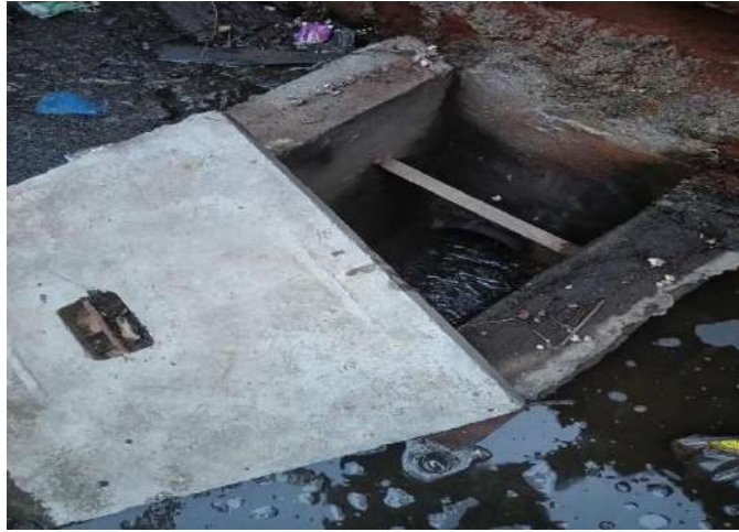
Chamber near ETP
