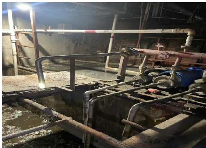
T- section provided on lifting pump.
