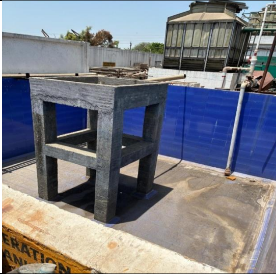
Old Aeration- (Spare now)
