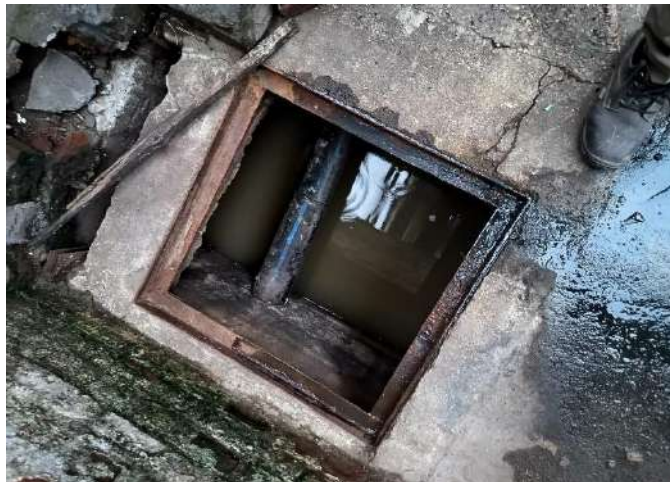
Storm water drain within premises.
